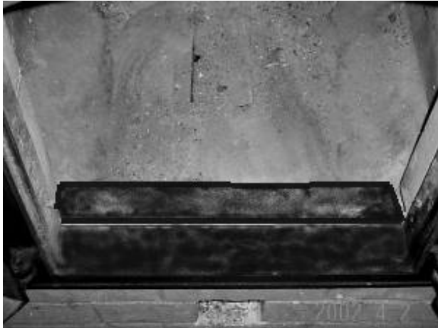
Figure 8 Air Bar is positioned and held in place with mortar at the ends. Refer to Figure 7 for dimensions.
