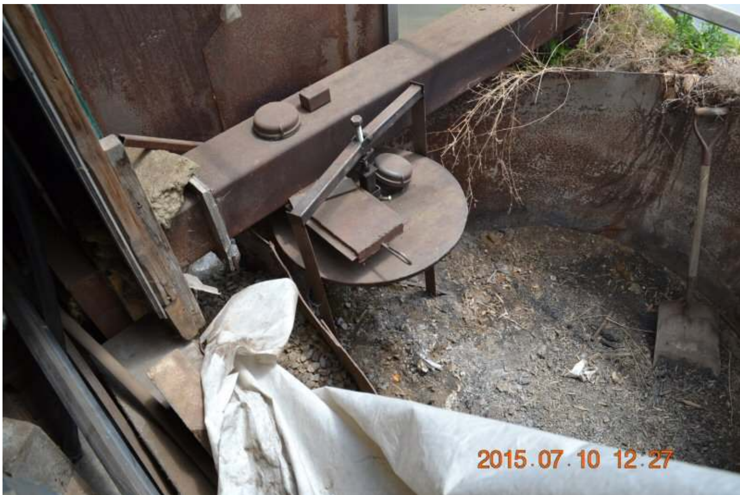
A prototype biochar takeoff. The square duct contains an airtight auger, that drops off the biochar into a drum.
