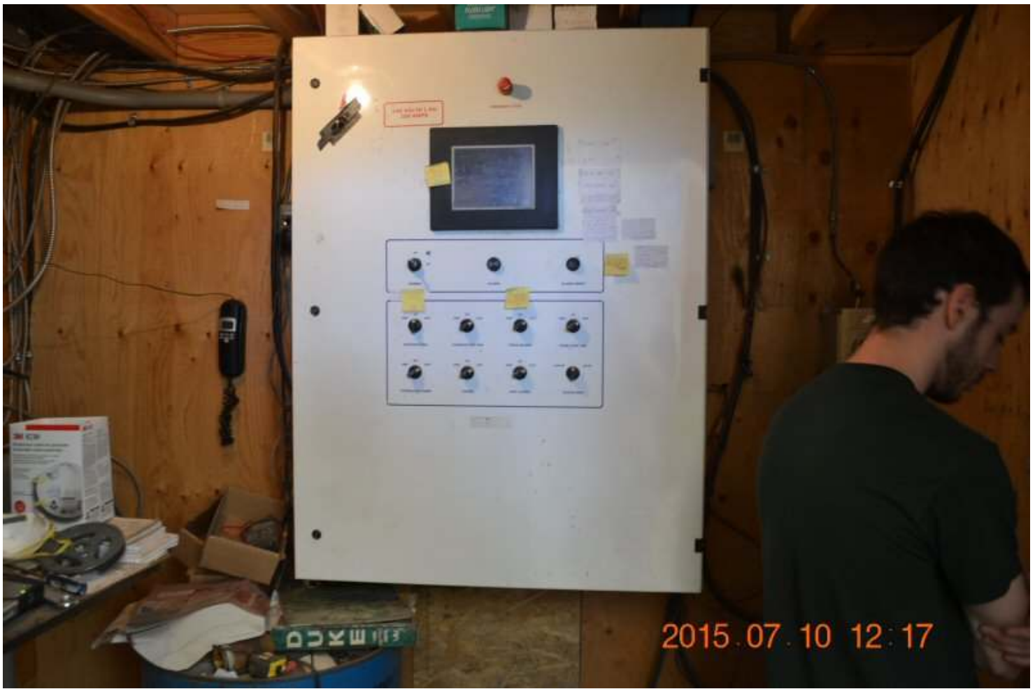
The PLC control system for the boiler.
