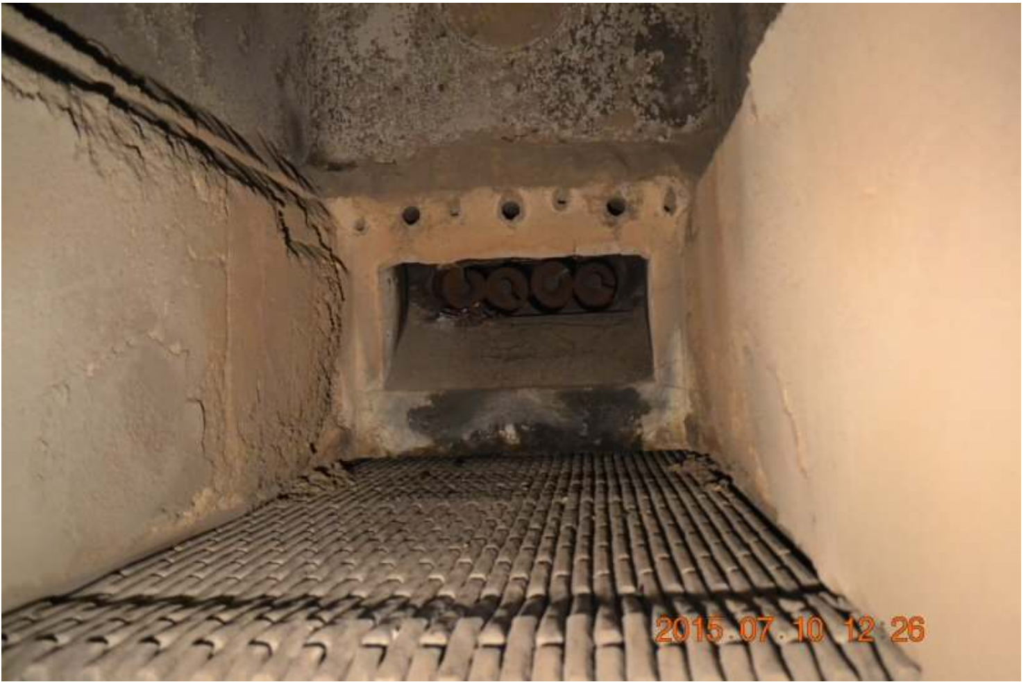
Four auger at the end are ganged in opposite directions, and feed the chips into the fire chamber.
