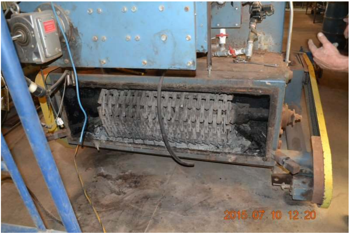
The moving chain grate.
