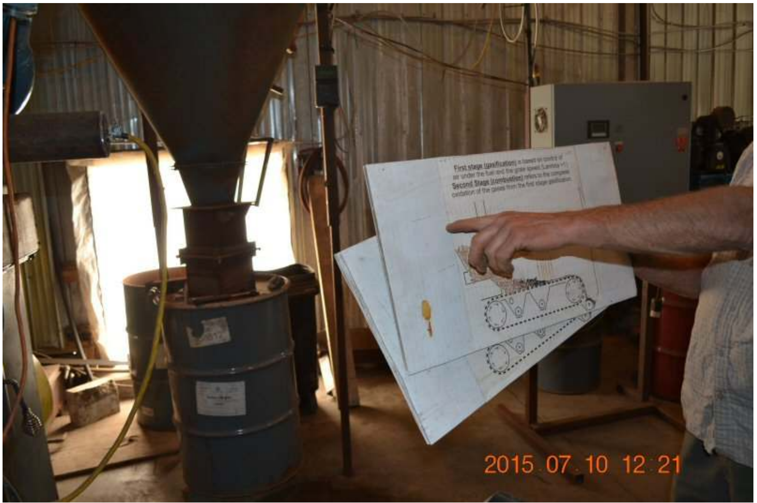
The boiler can be used to make biochar, by closing the primary air supply.
